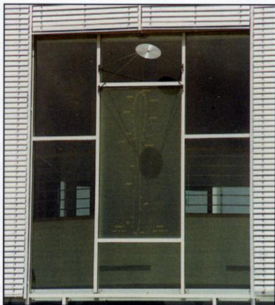
Figure 13: A view of the dial from the outside, which shows the finish on the gnomon disc and the gold lettering. A balcony at first floor level can be seen through the windows.
